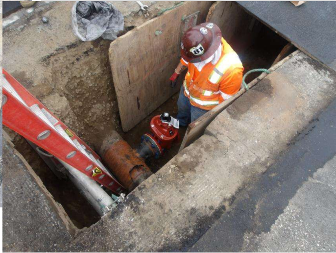
09/12/2024: Griffith Crew Installing 6" Gate Valves to FH Main Set for Tapping @ Sta. 339+98.
