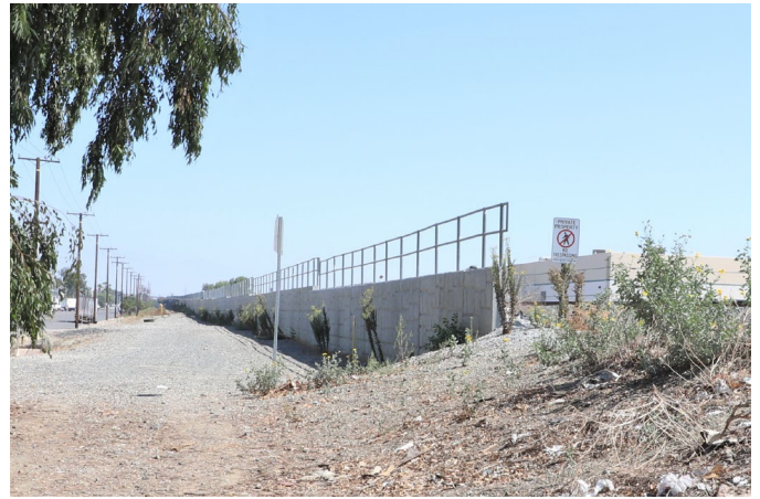
West end of wall associated with the modern grade separation on the north side of the SPRR tracks. Taken from the Guasti Road cul-de-sac approximately 500 feet west of N. Ponderosa Avenue. View east (9/30/22).
