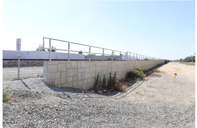
Wall associated with the modern grade separation along the north side of the SPRR tracks approximately 1,900 feet east of Milliken Avenue. Taken facing west-southwest (9/30/22).
