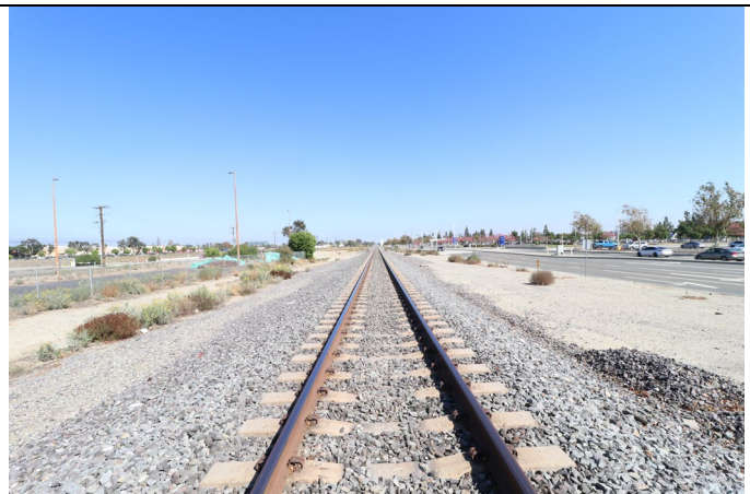
SPRR track facing east from a point approximately 2,500 feet west of Archibald Avenue (9/30/22). Ontario International Airport is to the south (right side of photo).
