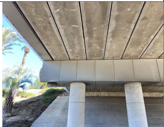
View of the crevices suitable for use by day roosting bats at the Union Pacific Railroad Bridge over Archibald Avenue (Structure 11).
