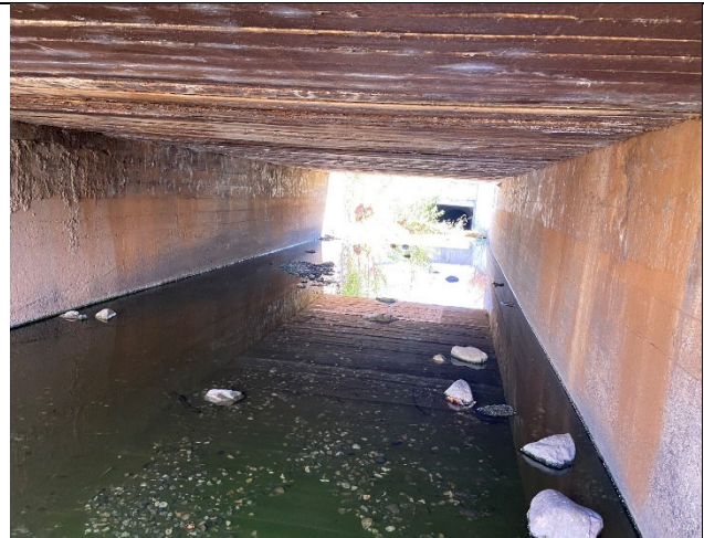
Representative view of the undersides of the timber bridge (Structure 9) spanning the drainage channel along the eastern edge of Turner Avenue. The entrance to the culvert beneath East Airport Drive is visible in the background.
