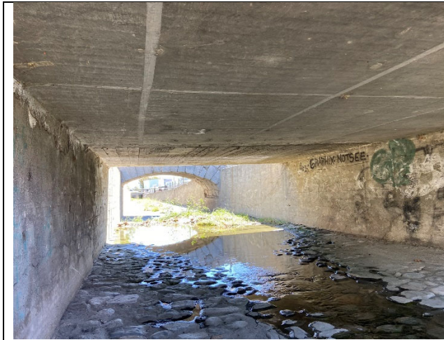
Representative view of the undersides of the concrete slab and stone arch bridges (Structures 5-8) spanning the drainage channel along the eastern edge of Turner Avenue.
