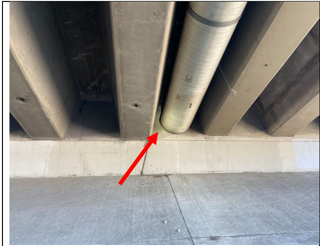
View of suitable day roosting habitat at the Milliken Avenue Overcrossing (Structure 1), which consists of weep holes and crevices around the pipe (red arrow). The bridge girders are suitable for night roosting.
