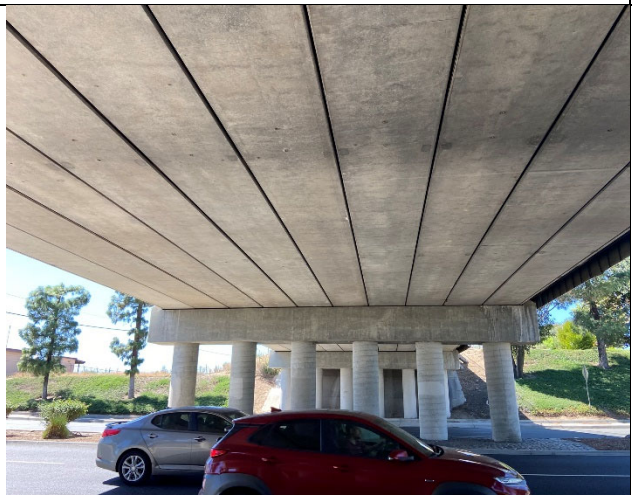
View of the crevices suitable for use by day roosting bats at the Union Pacific Railroad Bridge over Haven Avenue (Structure 4).
