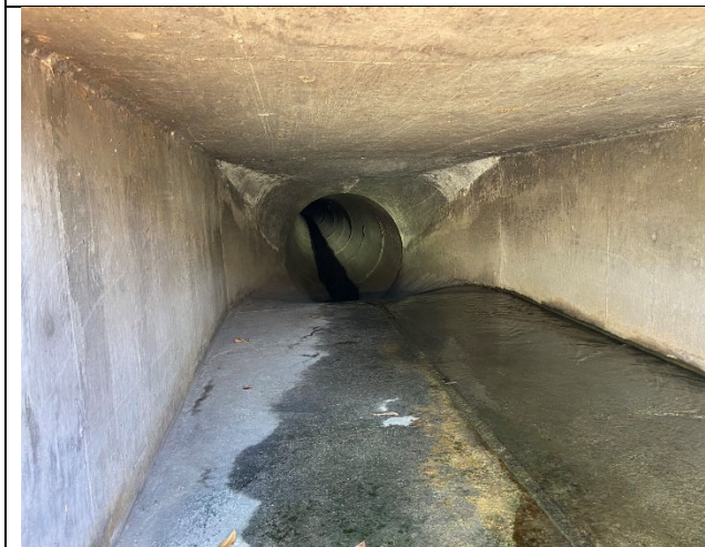
View of the culvert that carries the Turner Avenue drainage channel beneath East Airport Drive (Structure 10).
