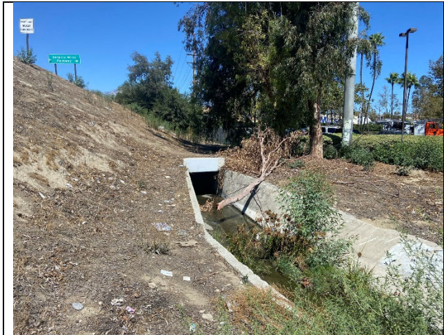
Small concrete box culvert adjacent to the Milliken Avenue Overcrossing and the foraging habitat along the drainage.
