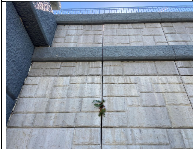
View of some of the crevices suitable for use by day roosting bats along the retaining wall at the Union Pacific Railroad Bridge over Milliken Avenue (Structure 3).
