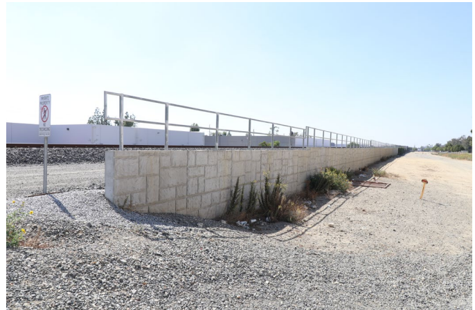
Wall associated with the modern grade separation along the north side of the SPRR tracks approximately 1,900 feet east of Milliken Avenue. Taken facing west-southwest (9/30/22).
