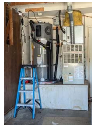
120V heat pump water heater installation in residence
