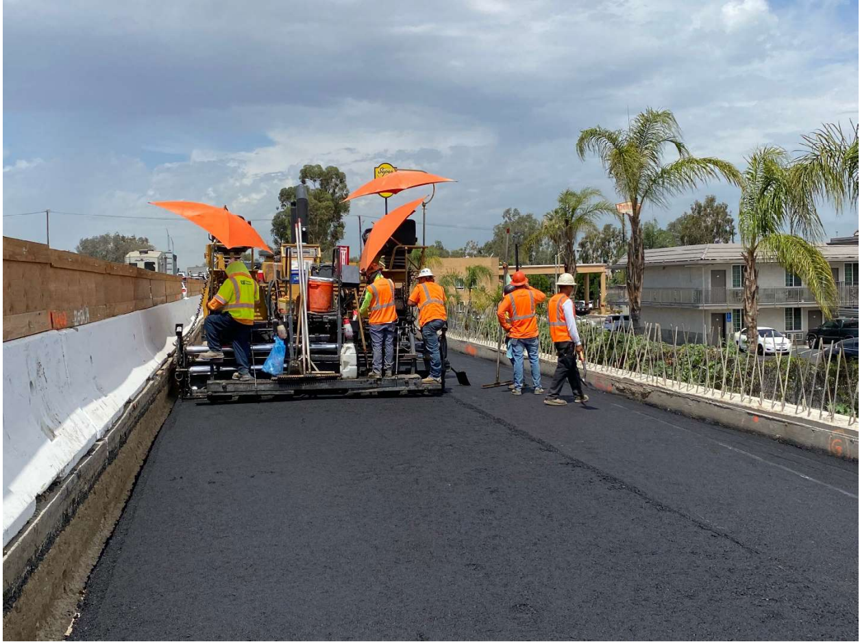
Paving crews install an asphalt base to the ramps at Interstate 10 and Alabama Street in Redlands.
