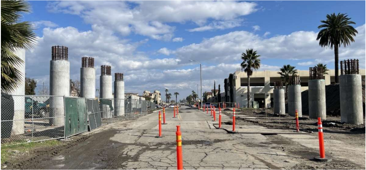
New columns rising out of the ground in preparation of the new bridge spanning over the Burlington Northern Santa Fe Railroad (BNSF) rail yard in San Bernardino.
