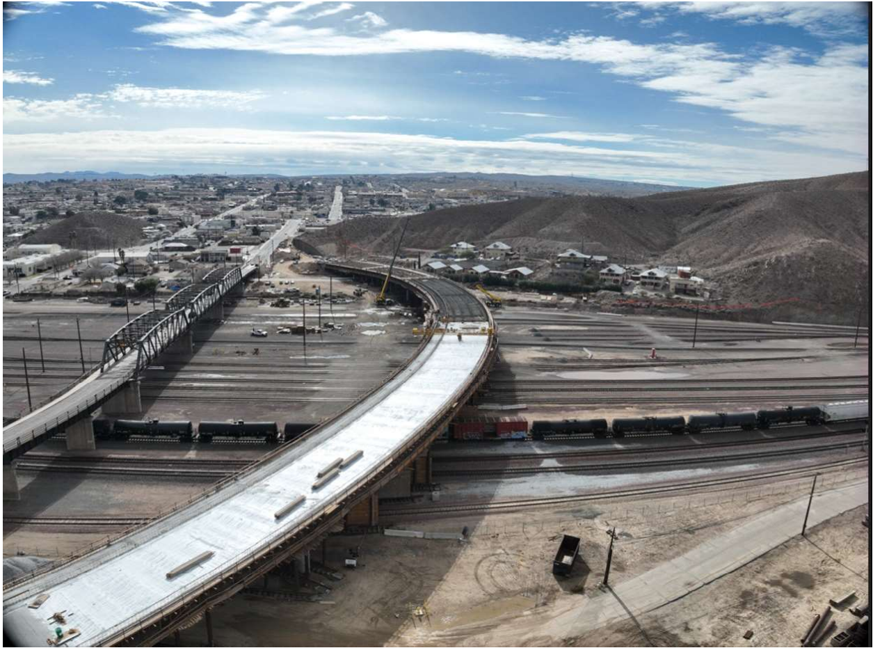
The City of Barstow can now see the progress of the new bridge spanning over the tracks in the southwest portion of the city. The old bridge is serving as a detour during the construction.
