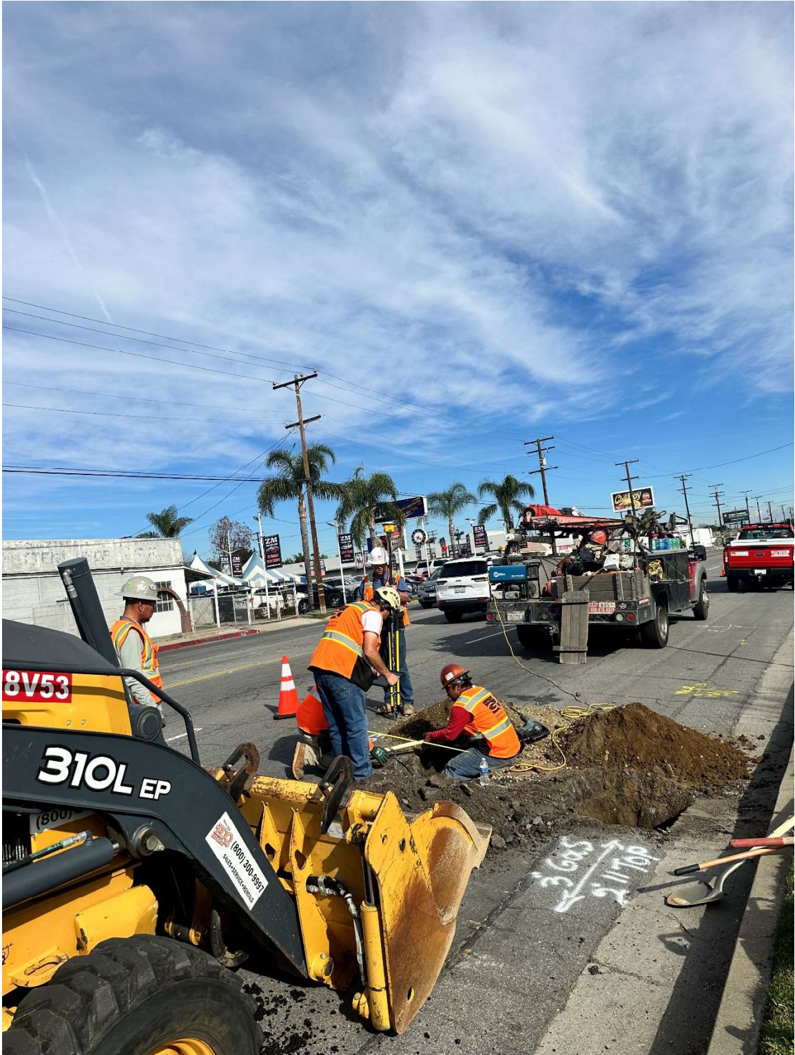
As the network evolves with the addition of new projects, utilities must be adjusted for the new configuration. Crews along the West Valley Connector Project corridor are seen here doing advance utility work.
